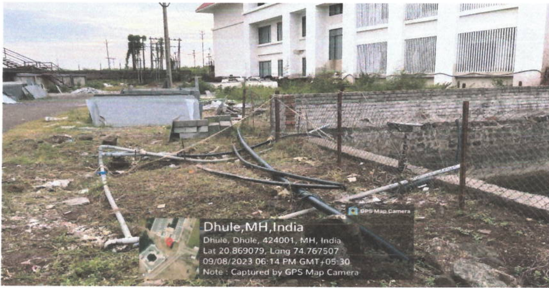
RWH drainage Pipes
